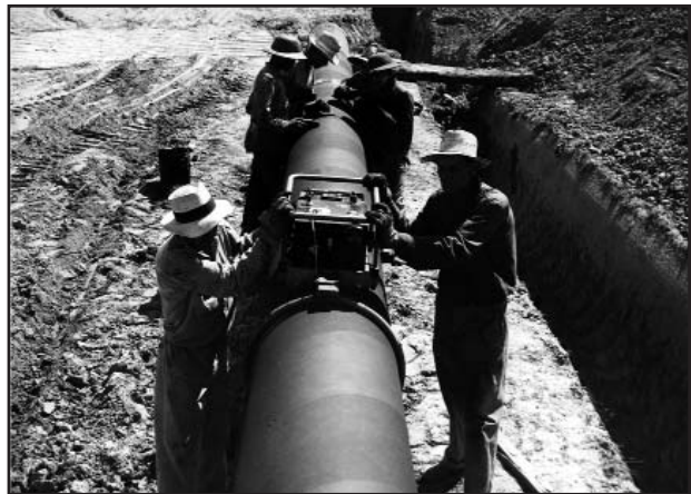
Inspecting the pipeline for holes before it is rolled into the trench. NARA 208-PRA-3-14-7128-20.
