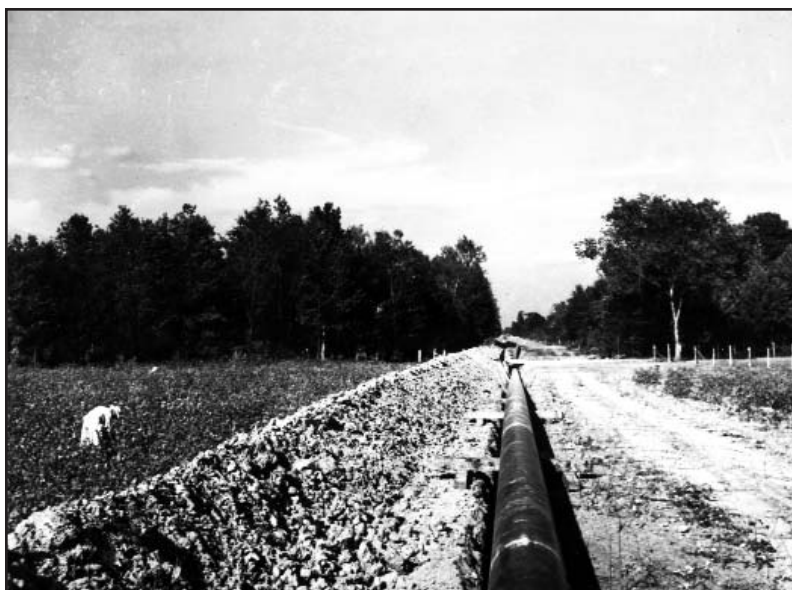
Little Rock, Arkansas, to Missouri-Arkansas state line, October 1942. War Emergency Pipeline from Longview, Texas, to Norris City, Illinois. Pipeline cutting through a cotton field. NARA 208-LU-37C-52.
