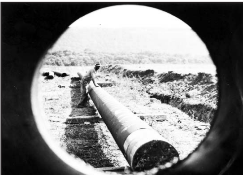
Viewed through a section of 24-inch pipe, a worker leans on a section of pipe ready for lowering into the ditch at right. NARA 208-LU-37C-34.
