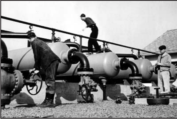
Utility men opening up oil filtering lines at WEP station near Eagle, Pennsylvania (November 1944). Parks-Standard Oil Company, New Jersey. NARA 208-LU-37C-16.
