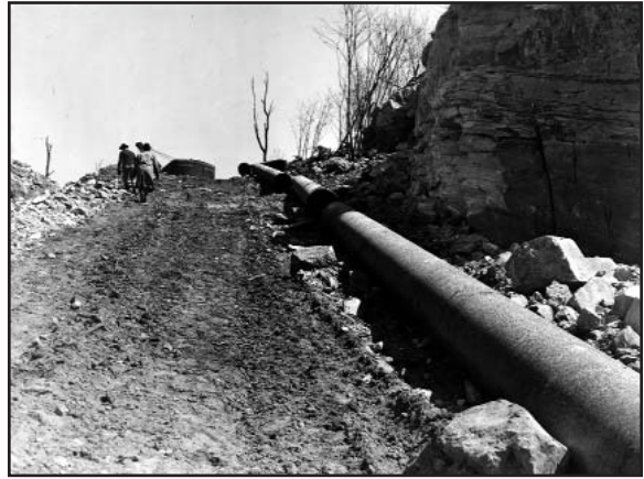
Sections of big inch pipe laid out on the pipeline right-of-way in Pennsylvania. NARA 253-CD-17-10.
