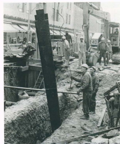
This I-beam smashed six telephone cables near the Stone Street office in 1970.
