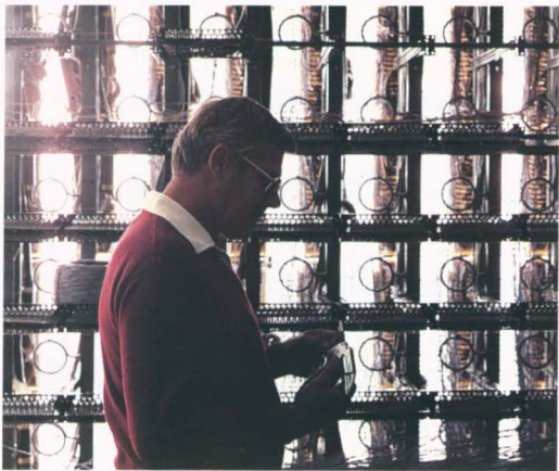
In another digital installation of the 1980's, switching technician Jim Waldorf connects cable pairs to the main distribution frame.
