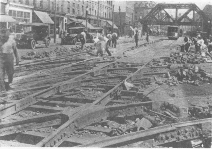
Laying new rails at State St. carbarn. Notice open touring automobiles and, in south, New York Central railroad bridge.
